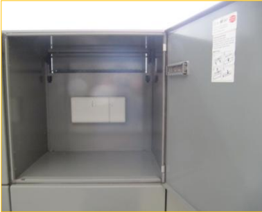
At the front ( under the opening )
